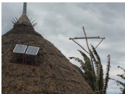
Left: The roof of a home in Maji with solar panels installed to provide electricity.
