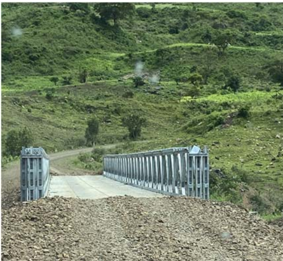
Getting a washed-out bridge replaced in a poor, rural corner of Ethiopia took all of Ato Markos’s skill, credibility, and persistence. When it got done, finally, trucks could carry supplies to the construction site!
